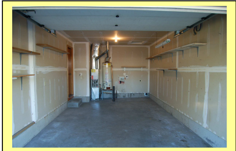
Washer/Dryer Hookups next to water heater
